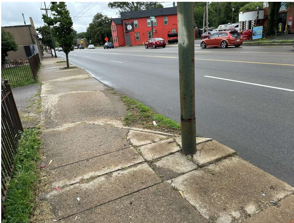
Figure 16. Weed growth, indicating poor drainage
